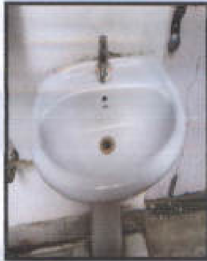
Water efficient Taps
